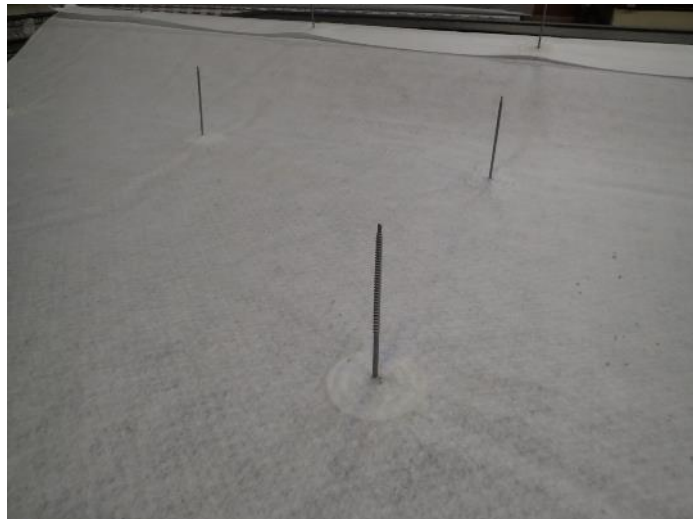
Photo 2 Detail of the failure mode.
